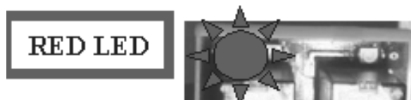
Relay Inside Ground Control Box
